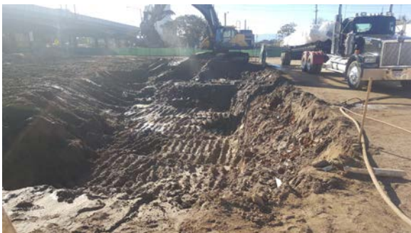
By end of day 2, mound was removed to one foot below grade, and areas of rows B and C were dug to 8 feet below grade.
