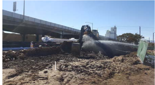
Wet methods included a water spraying nozzle on the excavator arm and a worker spraying from a hose.
