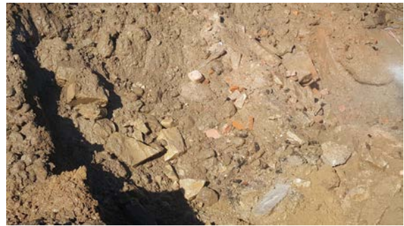
Building debris encountered during digging included concrete and brick.
