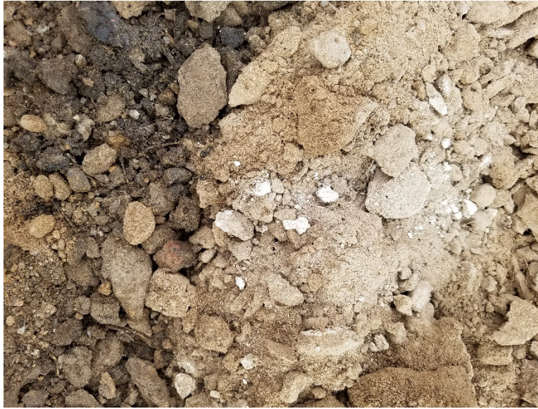
Non-ACM Plaster Debris
