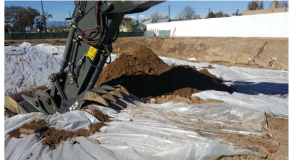
Potholing began in the area of the former mound, east side of the work area.
