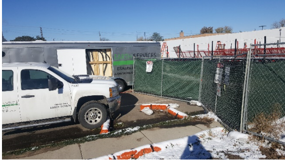
Three stage decontamination trailer with showers and negative air machine. Northeast end of work area.
