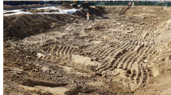
Grids 2A-6A, 2B-6B, 2C-6C are shown dug down to 8 feet below grade. Grids 2D-5D were excavated down to at least 1 foot below grade and covered with reinforced poly.
