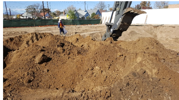
Potholed soil was clean of debris.
