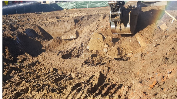
Debris – concrete foundation.
