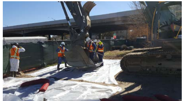
Gross removal of soil from bucket using hand tools conducted over a tarp.
