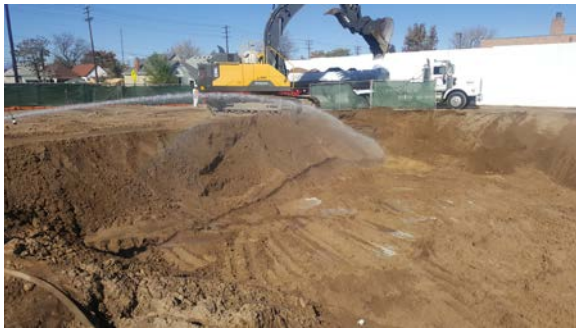
Digging continued west through grid 6A until all concrete foundation was removed.
