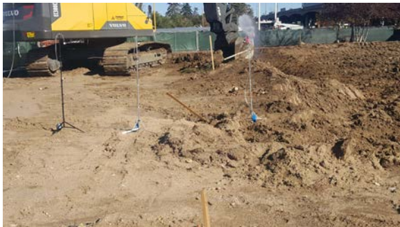
Western perimeter and western downwind sampling pumps.
