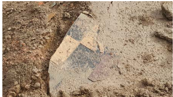
Debris- floor tile with mastic.
